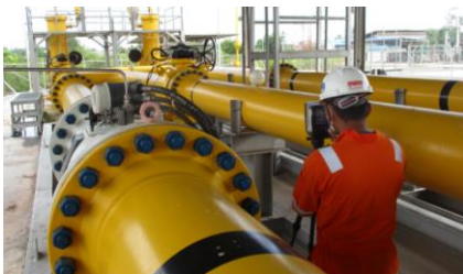
Gambar 5. Pipa Distribusi Gas Bumi
